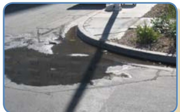
Casino Center Blvd. and Gass Ave. Facing south No sidewalk ramp, poor drainage
